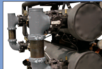
Evaporator manifold terminated in victaulic coupling.
