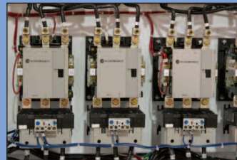
Close-up of the inside electrical panel
